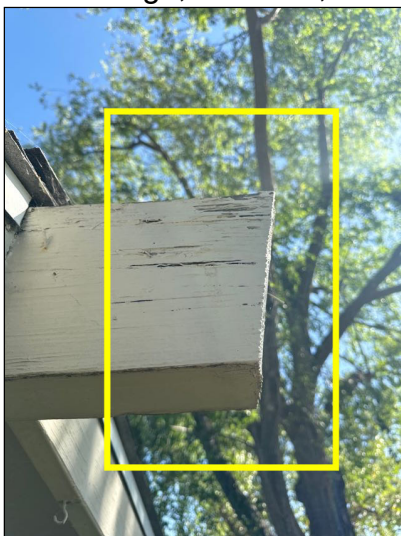
Moisture damage, wood rot, observed.
