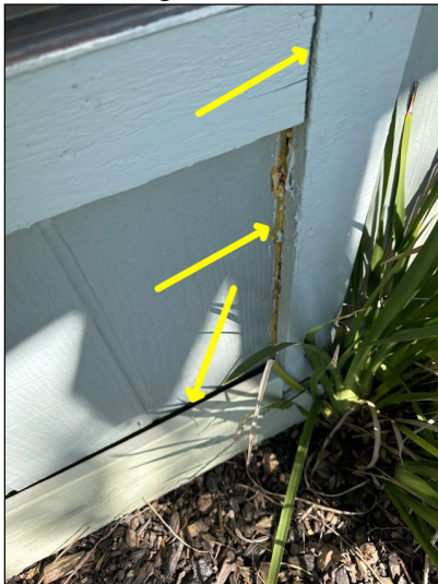
Moisture damage, wood rot, observed.
