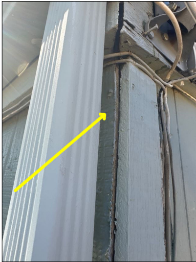
Missing trim should be replaced by a qualified contractor.
