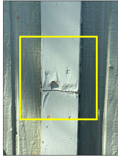
Moisture damage, wood rot, observed.
