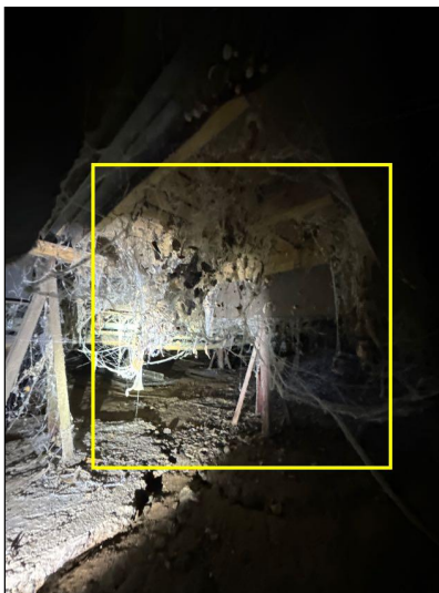
The dryer exhaust duct terminated in the crawlspace.
