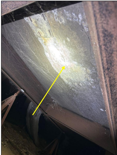
The sub floor had areas of localized advanced decay that appeared to be connected with plumbing fixture leakage.
