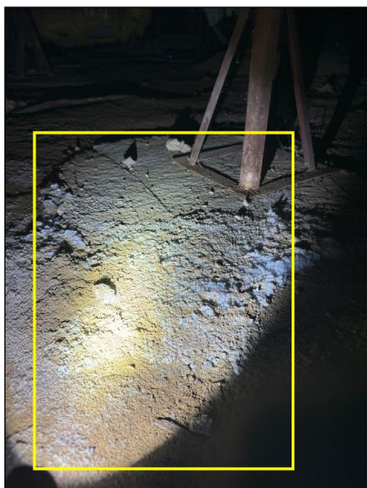
Soil in the crawlspace was visibly damp or wet.
