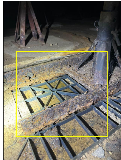
Steel beam girders supporting the floor structure in the crawlspace were supported by adjustable steel posts commonly called "screw jacks" on wood block.
