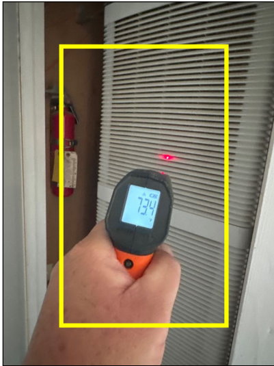
The differences in air temperature measured at supply and return registers fell within the acceptable range of between 14 and 22 degrees F.
