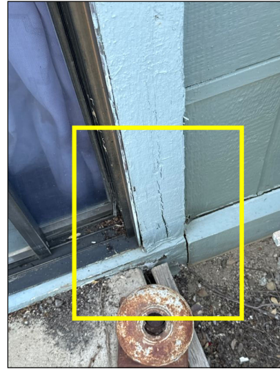
Moisture damage, wood rot, observed.
