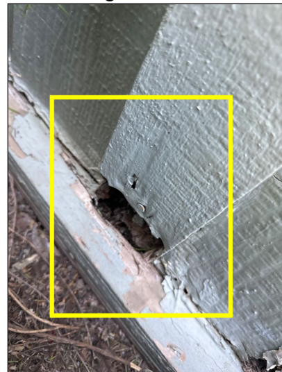
Moisture damage, wood rot, observed.
