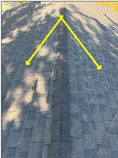
Monitor: Asphalt shingles covering some roof slopes exhibited severe deterioration and appeared to be at or near the end of their long-term service lives.
