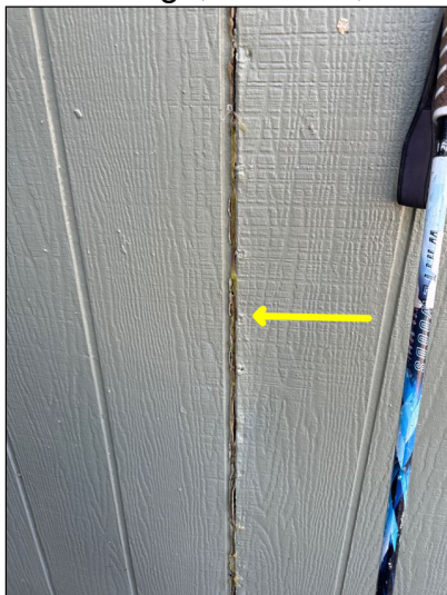
Routine Maintenance: Gaps at joints of the siding more than 1/4 inch (ca. 10 cm) should be sealed to keep unwanted moisture out. Recommend having joints sealed and painted. Continue to monitored as part of annual maintenance.
