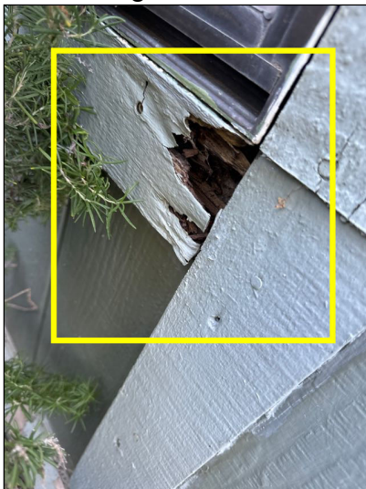
Moisture damage, wood rot, observed.
