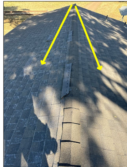
Monitor: Asphalt shingles covering some roof slopes exhibited severe deterioration and appeared to be at or near the end of their long-term service lives.
