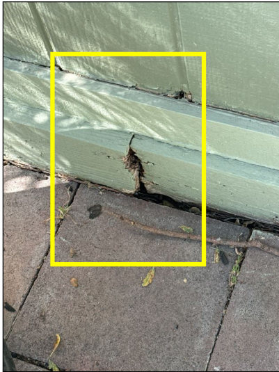
Moisture damage, wood rot, observed.
