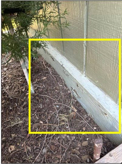
Moisture damage, wood rot, observed.
