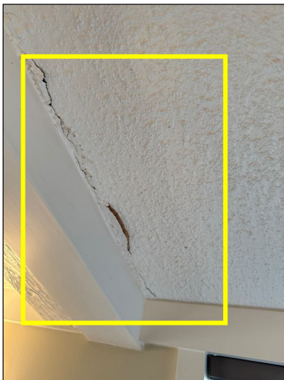
Monitor: Stains on the ceiling visible at the time of the inspection appeared to be the result of moisture intrusion.
