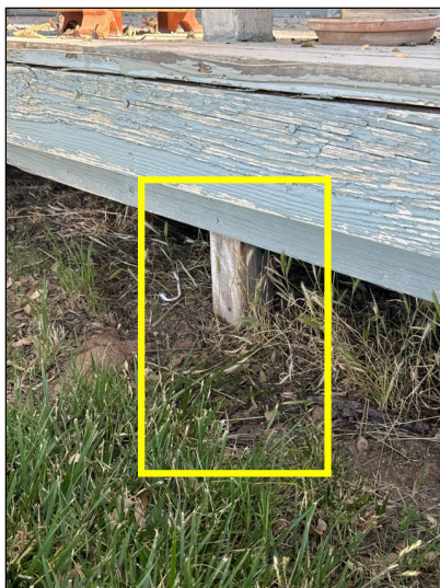
One or more posts supporting the deck had contact with soil at the time of the inspection.
