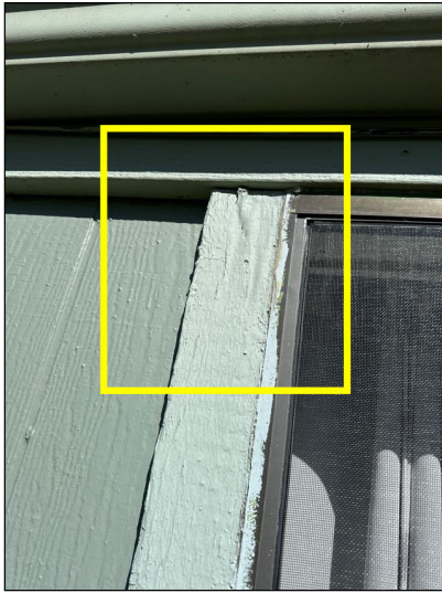
Moisture damage, wood rot, observed.
