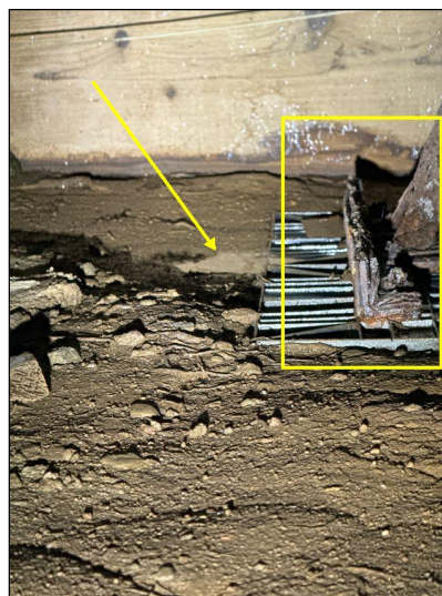
Water pooled in the crawlspace at the time of the inspection
