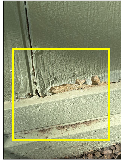
Moisture damage, wood rot, observed.
