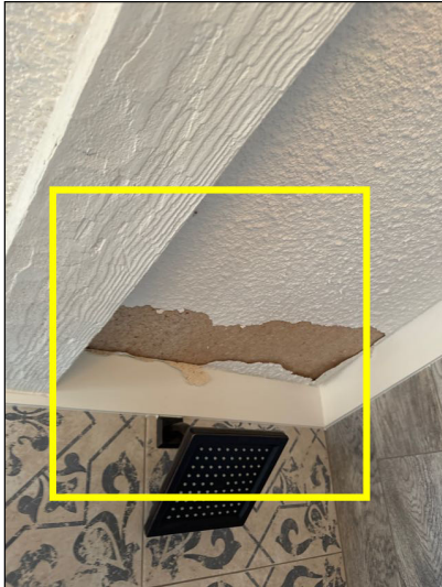
Monitor: Stains on the ceiling visible at the time of the inspection appeared to be the result of moisture intrusion.
