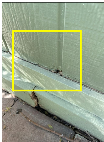
Moisture damage, wood rot, observed.
