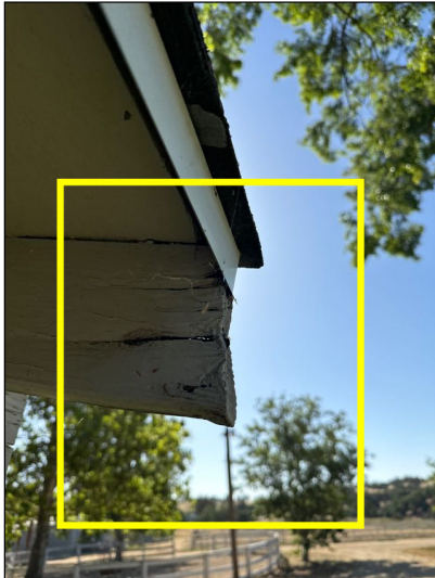
Moisture damage, wood rot, observed.
