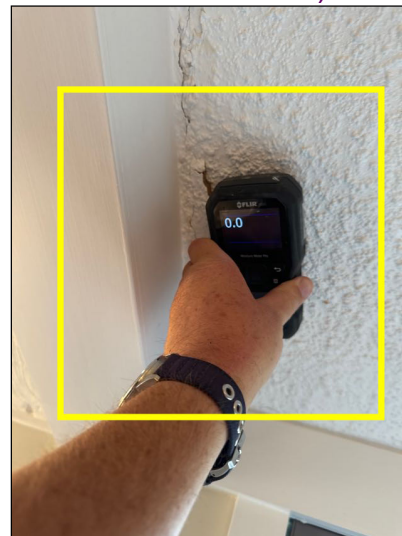
The moisture meter showed no elevated levels of moisture present in the stained areas at the time of the inspection (Normal moisture is considered between 5-12%)
