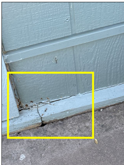
Moisture damage, wood rot, observed.
