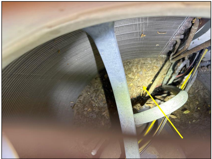
Monitor: The air-conditioner condenser unit had visible moderate of debris inside the cabinet.
