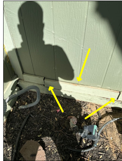
Maintenance Needed: Trim had gaps that should be filled with an appropriate sealant by a qualified contractor to help prevent moisture and insect entry.
