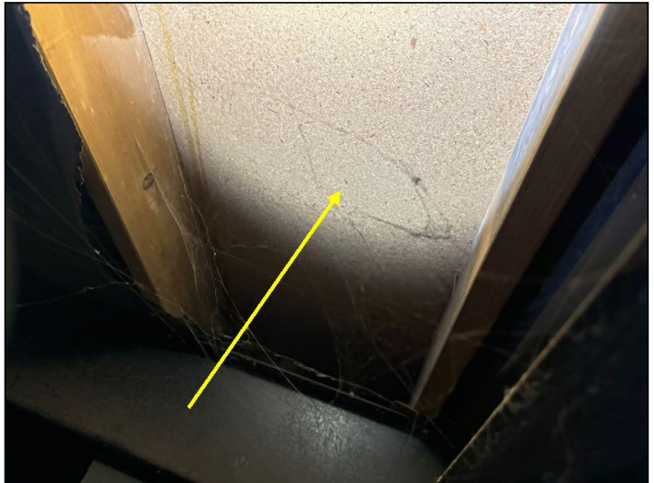
The floor structure consisted of particle board subfloor installed over conventional joists resting on the steel beam foundation.
