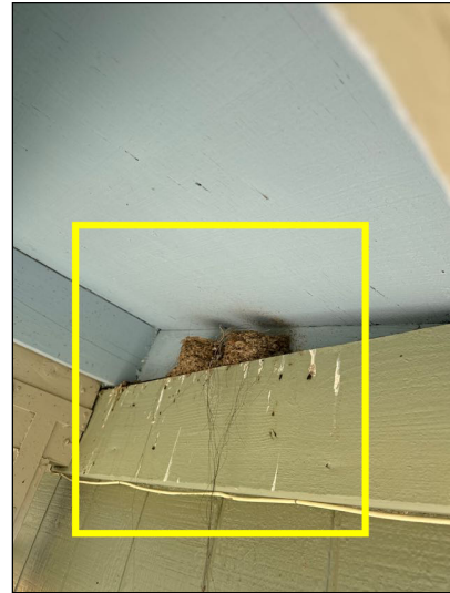
Monitor: Past Swallow nest evident under the soffits.
