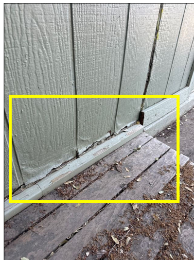
Moisture damage, wood rot, observed.
