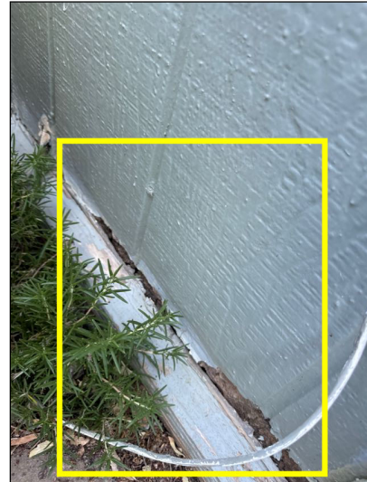
Moisture damage, wood rot, observed.
