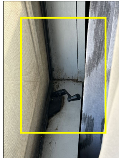
Windows sills in the home exhibited minor damage that appeared to be from moisture intrusion.
