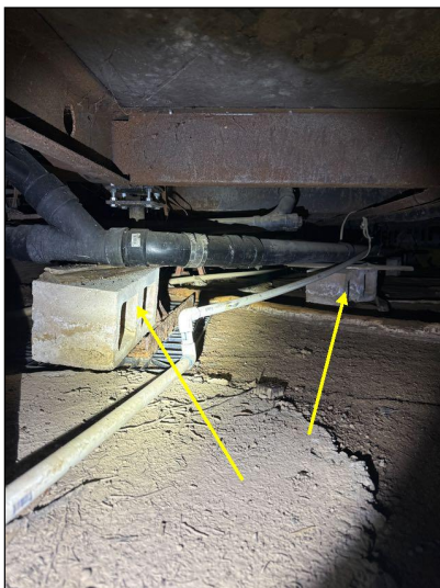
Plastic waste or drain pipes visible in the crawlspace were improperly supported.
