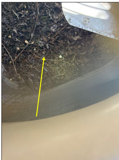
Monitor: The air-conditioner condenser unit had visible moderate of debris inside the cabinet.
