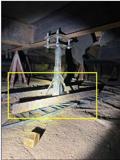
Steel beam girders supporting the floor structure in the crawlspace were supported by adjustable steel posts commonly called "screw jacks" on wood block.
