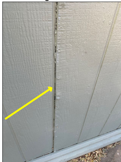
Routine Maintenance: Gaps at joints of the siding more than 1/4 inch (ca. 10 cm) should be sealed to keep unwanted moisture out. Recommend having joints sealed and painted. Continue to monitored as part of annual maintenance.
