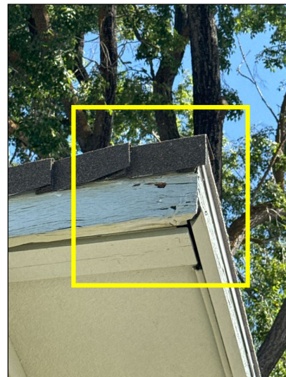
Moisture damage, wood rot, observed.
