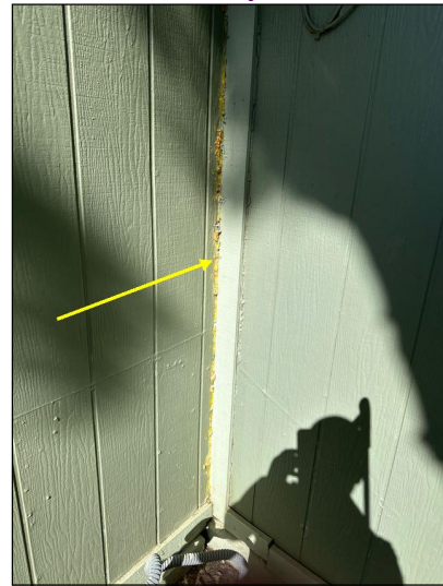
Maintenance Needed: Trim had gaps that should be filled with an appropriate sealant by a qualified contractor to help prevent moisture and insect entry.
