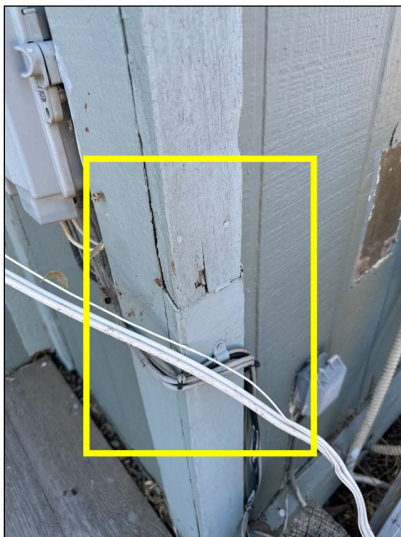
Moisture damage, wood rot, observed.
