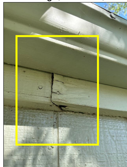
Moisture damage, wood rot, observed.
