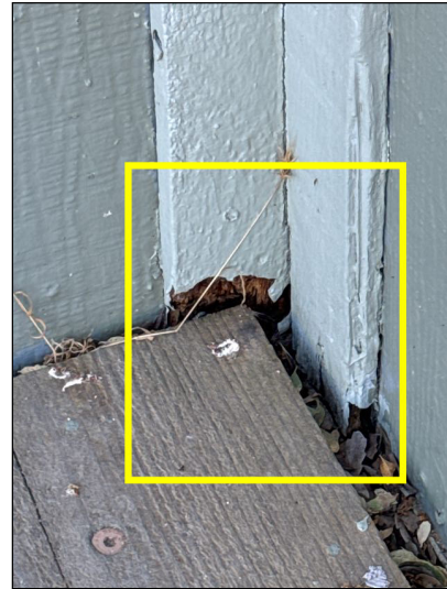
Moisture damage, wood rot, observed.
