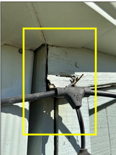
Moisture damage, wood rot, observed.
