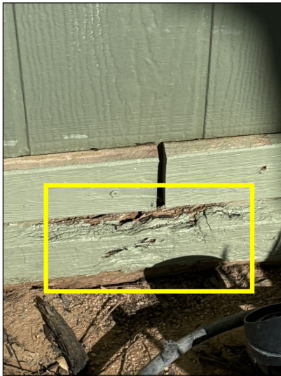
Moisture damage, wood rot, observed.
