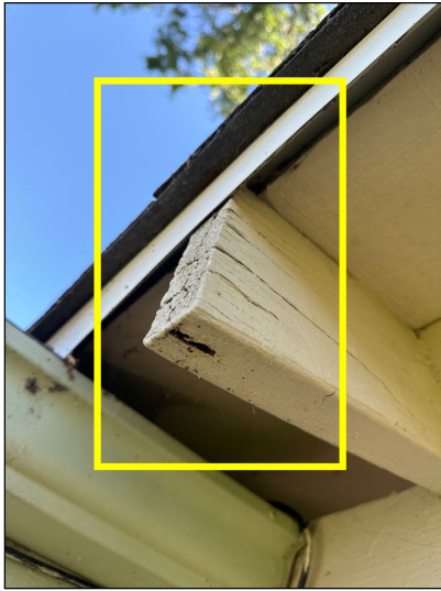
Moisture damage, wood rot, observed.
