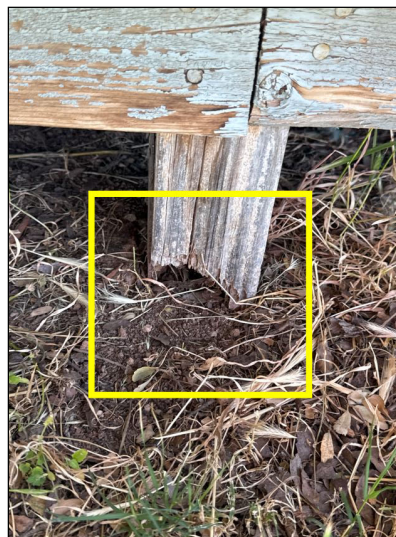
Foundation piers supporting the porch appeared to be unstable at the time of the inspection.
