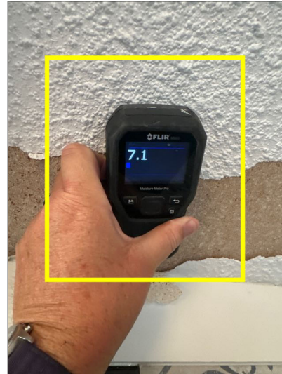
The moisture meter showed no elevated levels of moisture present in the stained areas at the time of the inspection (Normal moisture is considered between 5-12%)
