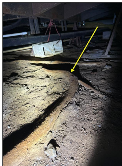
Tree roots growing under the home
