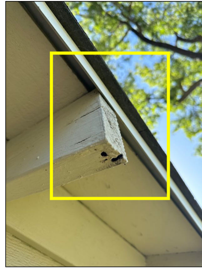
Moisture damage, wood rot, observed.
