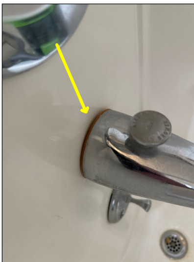
The tub faucet in this bathroom not flush to wall.
