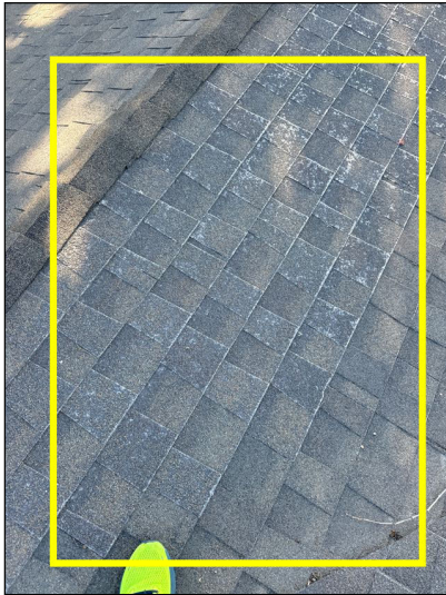
The asphalt composition shingles covering the roof of this home showed moderate deterioration that appeared to be commensurate with the age of the roof.
