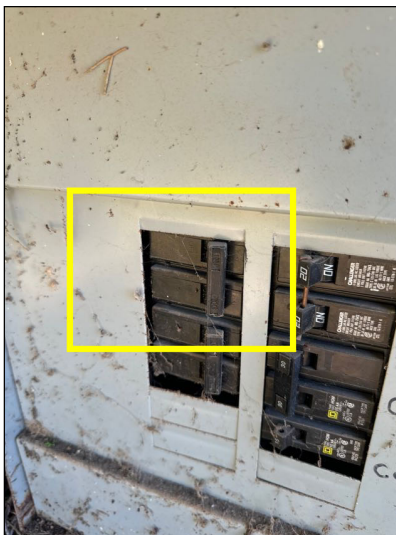
Main electrical shut off to the home
