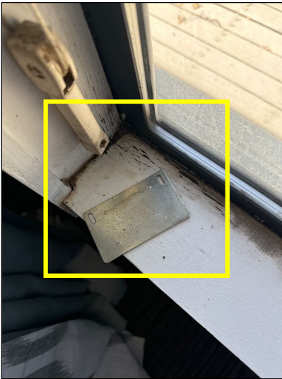
Windows sills in the home exhibited minor damage that appeared to be from moisture intrusion.
