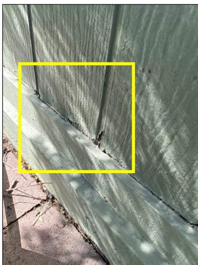
Moisture damage, wood rot, observed.
