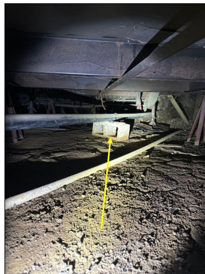
Plastic waste or drain pipes visible in the crawlspace were improperly supported.
