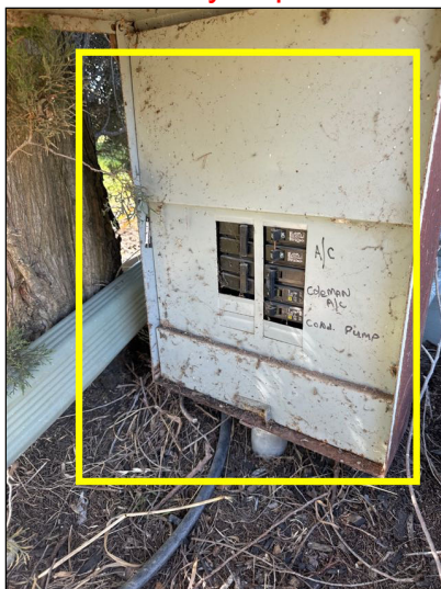
Main electrical service panel to the home.
