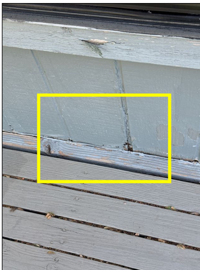
Moisture damage, wood rot, observed.
