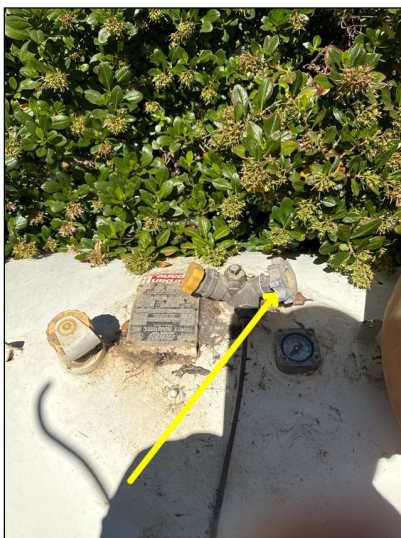
Main shut off to the liquid propane tank
