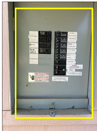
Sub panel to the home
