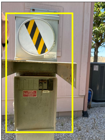
Main electrical service pedestal to the home.
