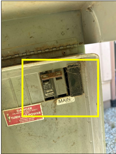
Main electrical shut off at the electrical pedestal.
