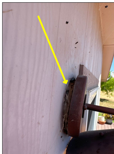
Exterior lighting was loose to the wall and could expose electrical components to moisture intrusion.
