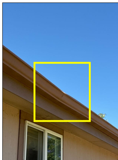
The gutters were bent or damaged in areas.
