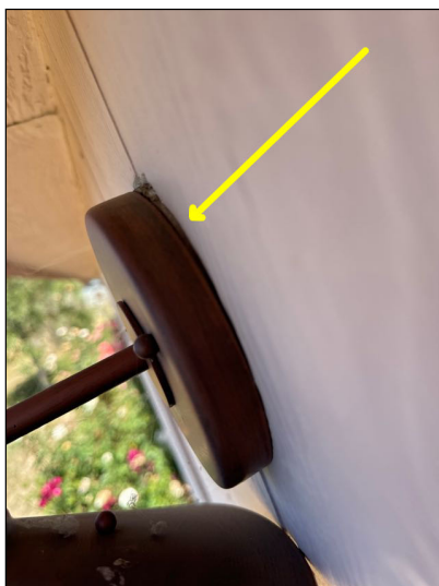
Exterior lighting was loose to the wall and could expose electrical components to moisture intrusion.
